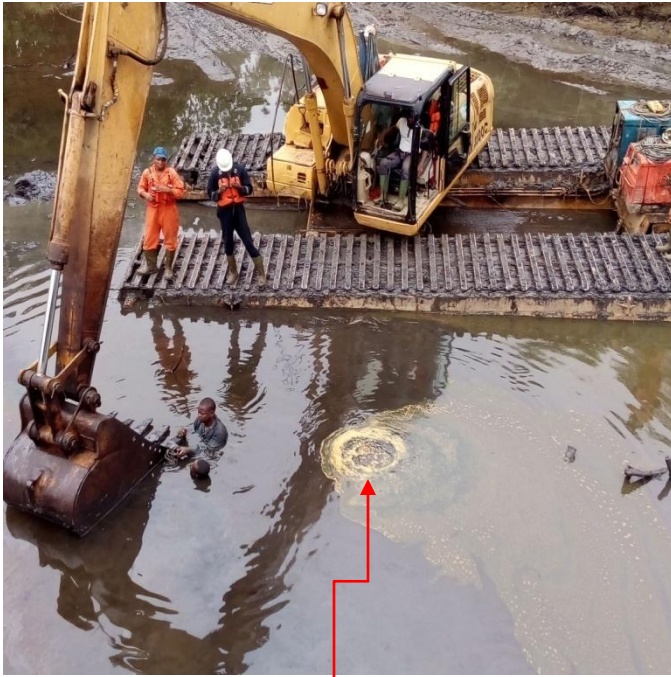
Fig A: Spill point just before excavation
